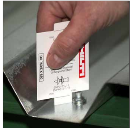
Checking the standoff of an ENP2 roof deck fastening with a plastic gauge
