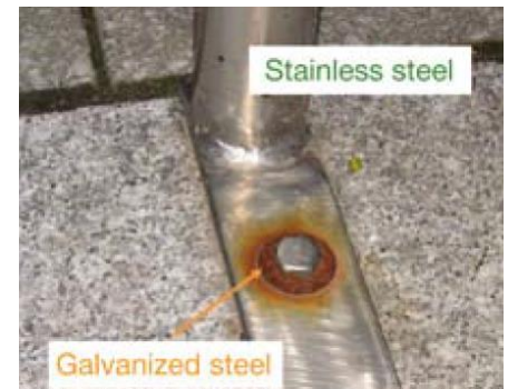
This is a typical case of contact corrosion. Zinc-plated carbon steel (washer) and stainless steel (screw and part) were used together. The surface area of the more noble metal – the stainless steel – is larger, causing strong corrosion of the washer.
