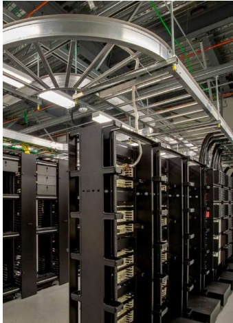
Support cable tray
